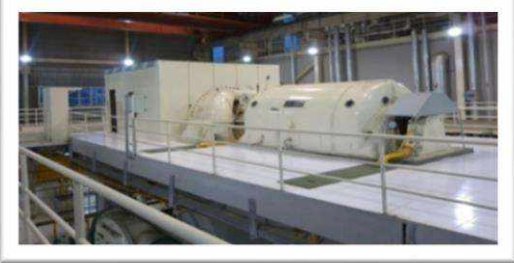
POWER PLANT Capacity : 15 MW Turbine & 2 Boiler x 40 ton
