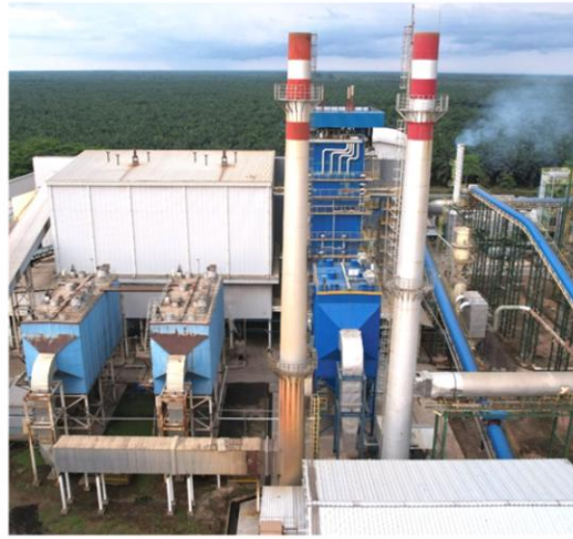
POWER PLANT Kapasitas : 30 MW Turbine, 2 Boiler x 40 ton & 1 CFB Boiler x 80 ton
